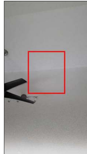
Evidence of previous repair observed. Unable to determine the effectiveness of the repair.
