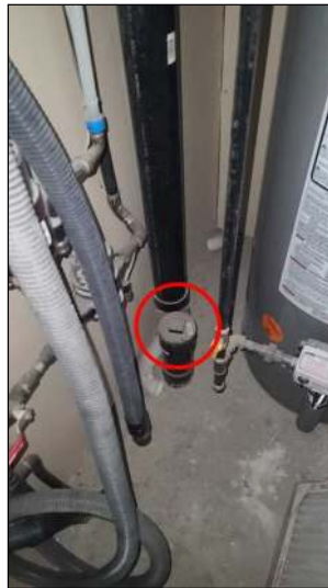
Main cleanout is accessible
