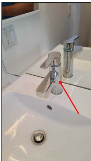
Faucets are loose. Recommend securing to ensure proper function
