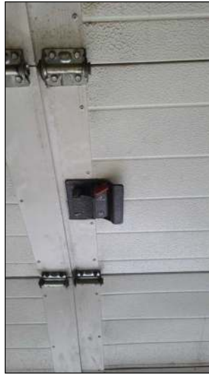
The man door latch is not functional and should be serviced
