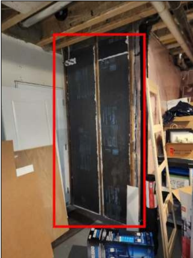
Any visible spray foam or polystyrene insulation needs to be fire protected to protect against any off gassing in the case of a fire. There are multiple gaps in the joist ends in the basement. Have a contractor evaluate and service as needed.
