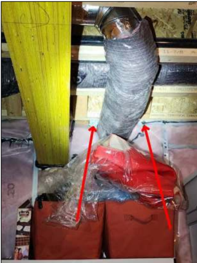
Any visible spray foam or polystyrene insulation needs to be fire protected to protect against any off gassing in the case of a fire. There are multiple gaps in the joist ends in the basement. Have a contractor evaluate and service as needed.
