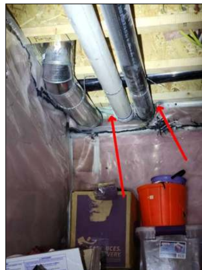
Any visible spray foam or polystyrene insulation needs to be fire protected to protect against any off gassing in the case of a fire. There are multiple gaps in the joist ends in the basement. Have a contractor evaluate and service as needed.
