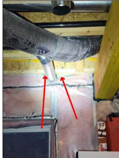
Any visible spray foam or polystyrene insulation needs to be fire protected to protect against any off gassing in the case of a fire. There are multiple gaps in the joist ends in the basement. Have a contractor evaluate and service as needed.
