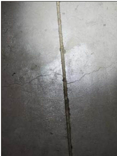
Common cracks noted.
