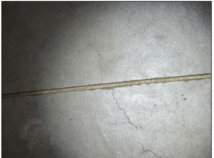
Common cracks noted.
