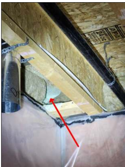
Any visible spray foam or polystyrene insulation needs to be fire protected to protect against any off gassing in the case of a fire. There are multiple gaps in the joist ends in the basement. Have a contractor evaluate and service as needed.
